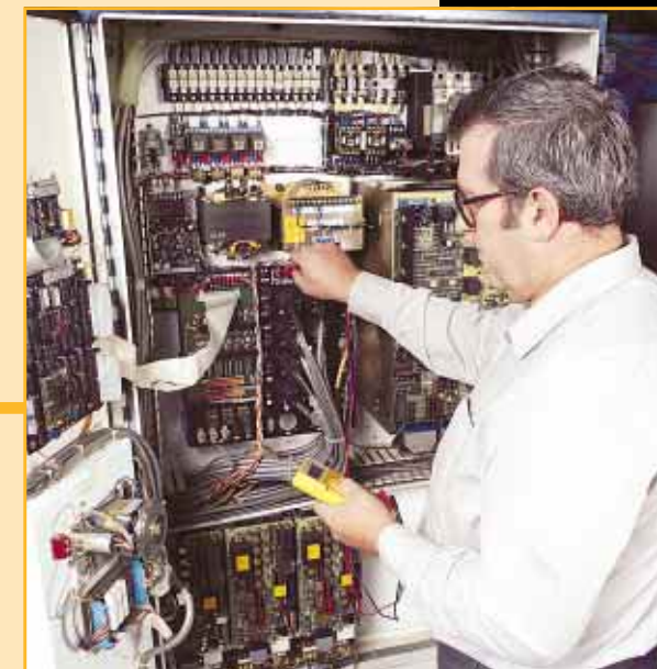
controls and other motor control systems.
